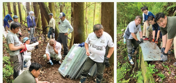
Installation of metal plates on local aqueducts in collaboration with the local neighborhood association
