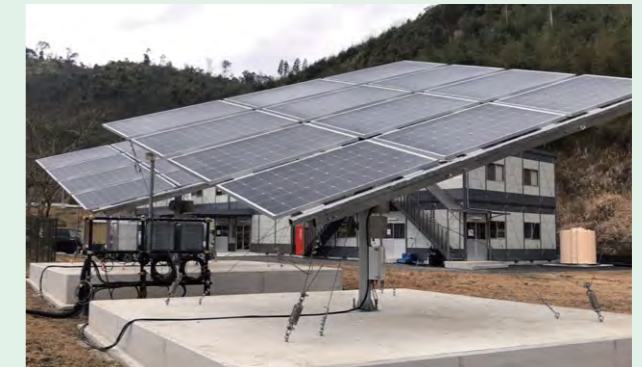
Sun-tracking solar power generation system
