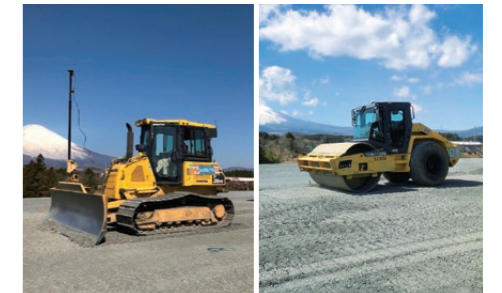
Utilization of machine-control (automation and remote control) bulldozers and rollers equipped with a banking/landfill 3D management system
