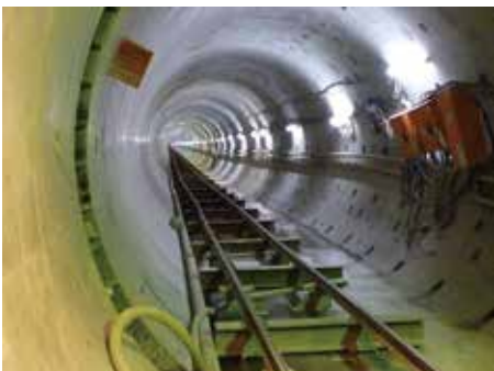
Temporary LED lighting at sites
