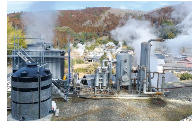
Power generation plant overview
