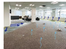
Yukarela air-conditioning system While transmitting heat to the OA flooring by flowing air under the floor, solar radiation load is reduced by releasing it into the office from recirculating ports near windows
