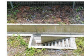
Gutter staircase for small animals (Kanto Civil Engineering Regional Headquarters, Minami Koma Worksite Office)
