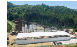
Concrete plant painted in natural colors (North Japan Regional Headquarters, Kawauchisawa dam Site Office)
