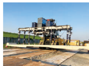
Full-scale transport and installation experiment using a large forklift and dedicated installation equipment
