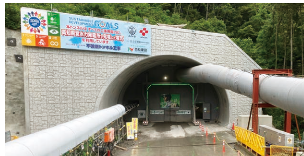
Tunnel construction site using renewable energy for 100% of construction power (Shikoku Branch, Fubahara Tunnel Branch Office)
