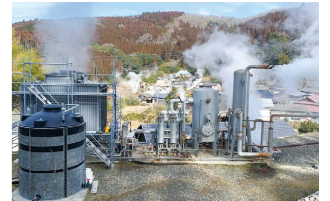
Power generation plant overview
