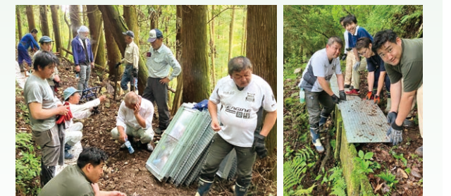
Installation of metal plates on local aqueducts in collaboration with the local neighborhood association
