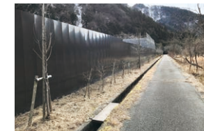
Temporary fencing using earth tones (Kanto Civil Engineering Regional Headquarters, Minami Koma Worksite Office)
