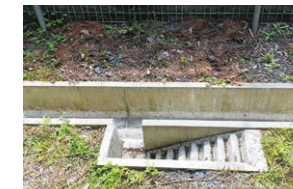
Gutter staircase for small animals (Kanto Civil Engineering Regional Headquarters, Minami Koma Worksite Office)
