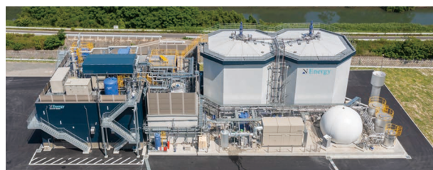
Western Kumamoto Biogas Power Plant
