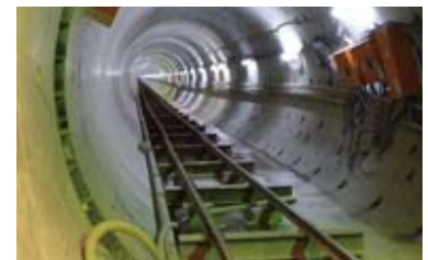
LED lighting inside shield tunnel construction sites
