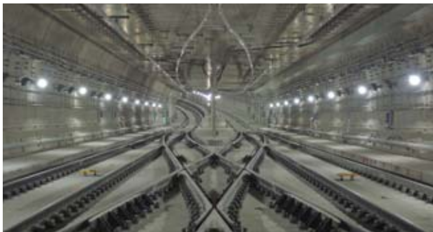
Hong Kong Subway South Island Line Nam Fung Tunnel and Ventilation Tower Construction
