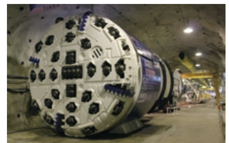
Tunnel Boring Machine for Pahang-Selangor Raw Water Transfer Project, Lot 1-1, Water Transfer Tunnel and Related Works, Malaysia
