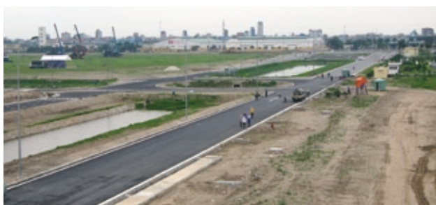
Construction and Completion of Infrastructure Works under Second Stage of Thang Long Industrial Park II (Vietnam)
