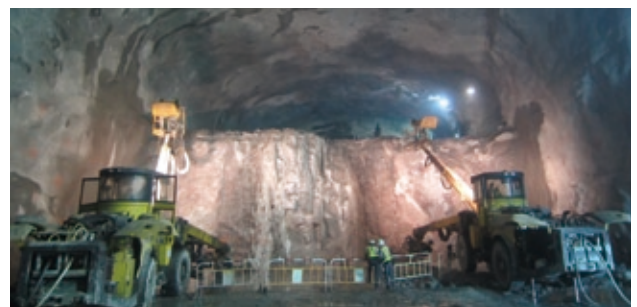
Construction of Large Cavern for Sai Ying Pun Station, C704 (Hong Kong)
