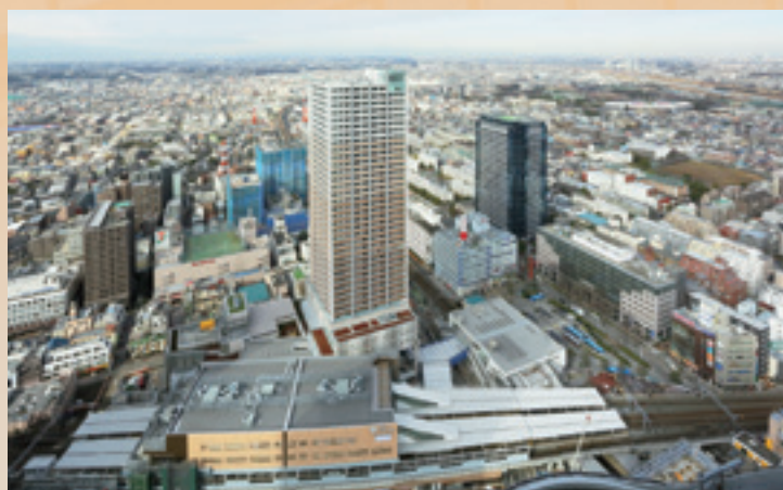
Complex Building Construction, West Town Area of Musashikosugi Station South Exit Area, 1st Class Urban Area Redevelopment Plan
