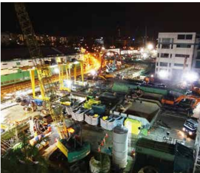
Contract 929A Construction and Completion of Tunnels between Ubi and Kaki Bukit Station and Reception Tunnels for Down Town Line 3
