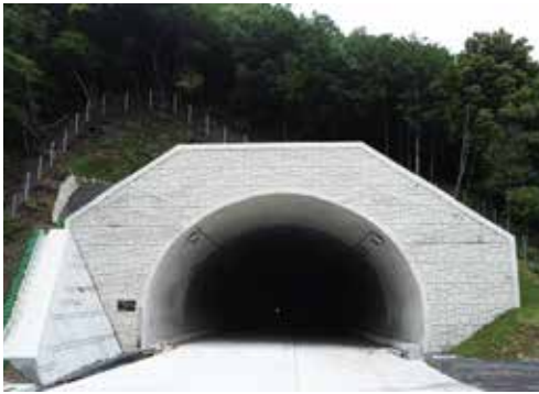
Kongoji Tunnel Construction, Nachikatsuura Road Completed: January 2015 Location: Nachikatsuura-cho, Higashimuro-gun, Wakayama Prefecture
